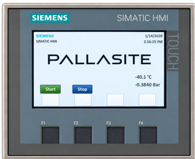
Siemens HMI — Integrated System Control
